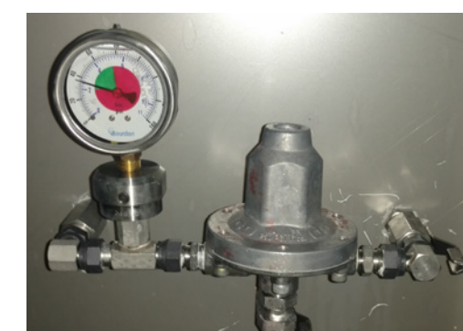
Using Fluid Pressure and Fluid Flowrate control at the Cleaning station:
