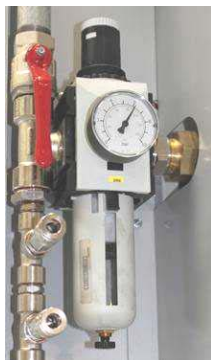
Compressed air supply
