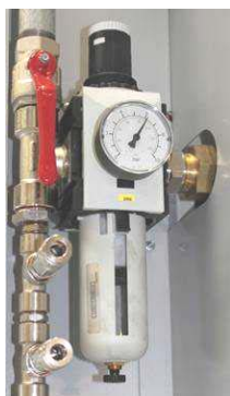
Compressed air supply
