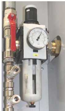
Compressed air supply
