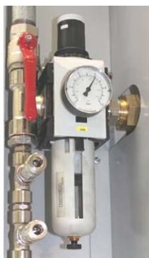
Compressed air supply
